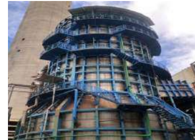
Power Plant Desulfurization
