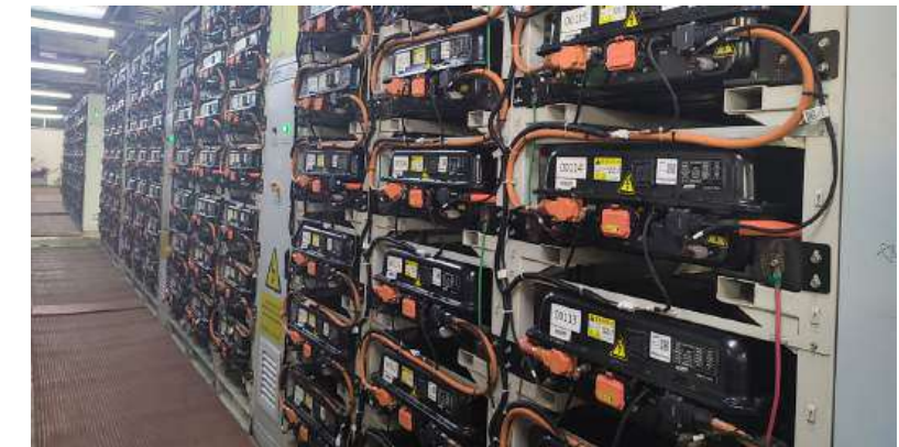
Hot-rolled Lithium Battery Energy Storage Project
