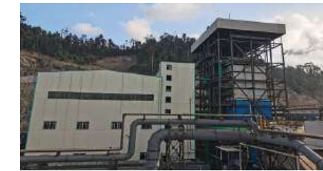
PT.DSI 1*150MW Power Plant
