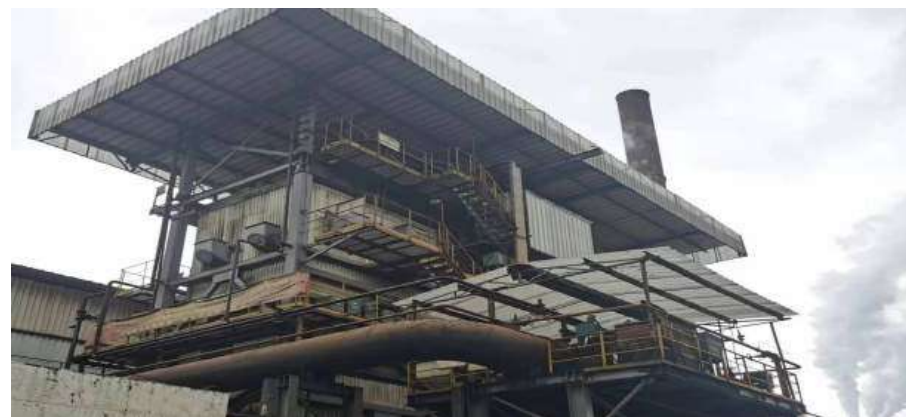
PT.TSI-7 MW Power Plant
