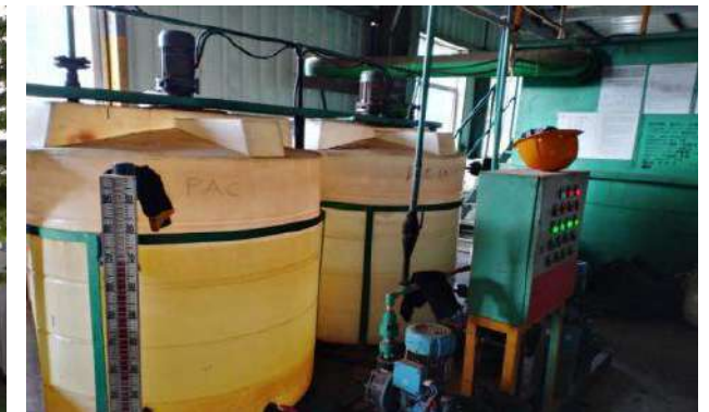
Domestic Sewage Purification Treatment Plant
