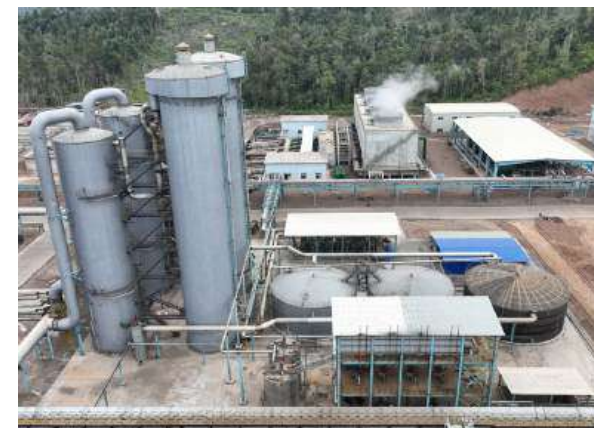
Gas Purification and Hydrogen Disulfide Removal System
