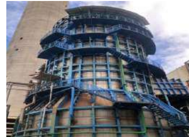
Desulfurisasi power plant
