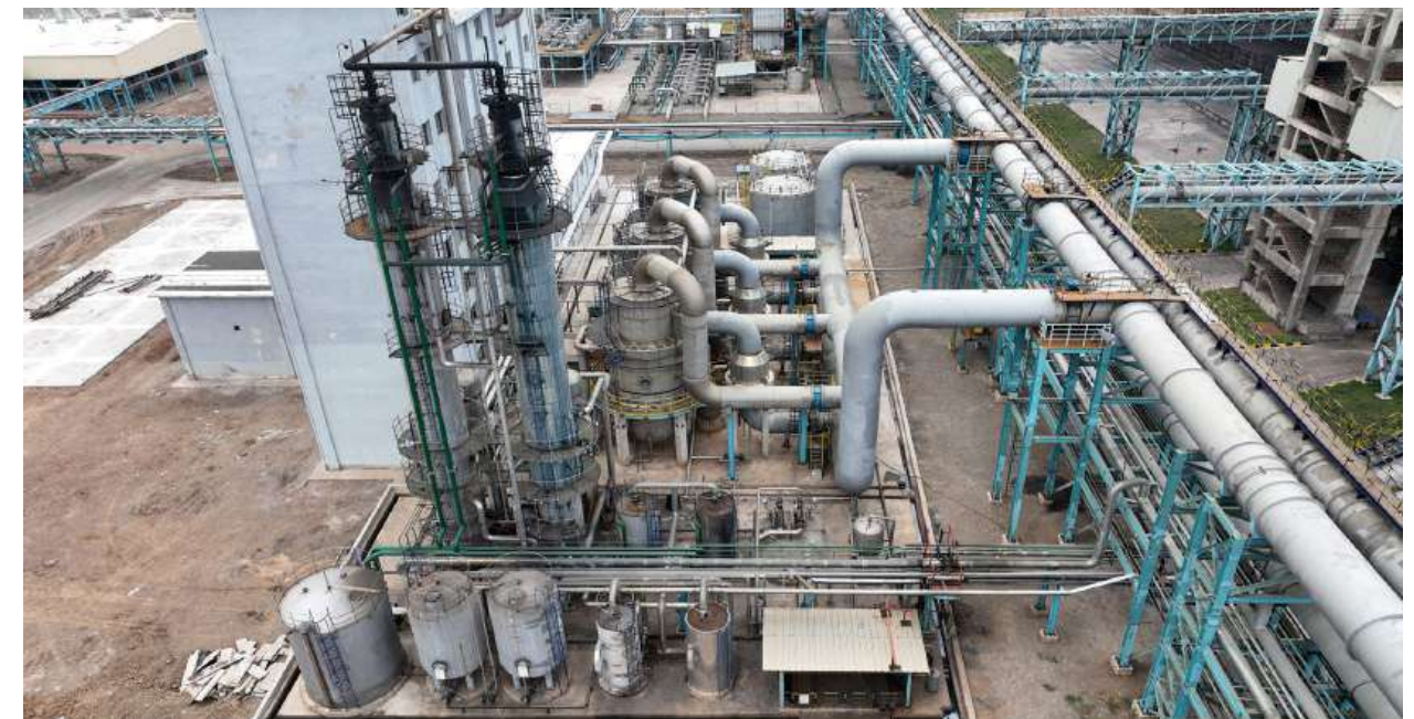
Production Wastewater Treatment Plant - Ammonia Evaporation System
