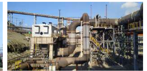
PT.DSI TRT Residual Pressure Power Plant
