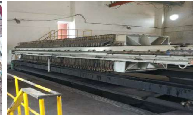
Production Wastewater Filter Press Treatment and Recycling
